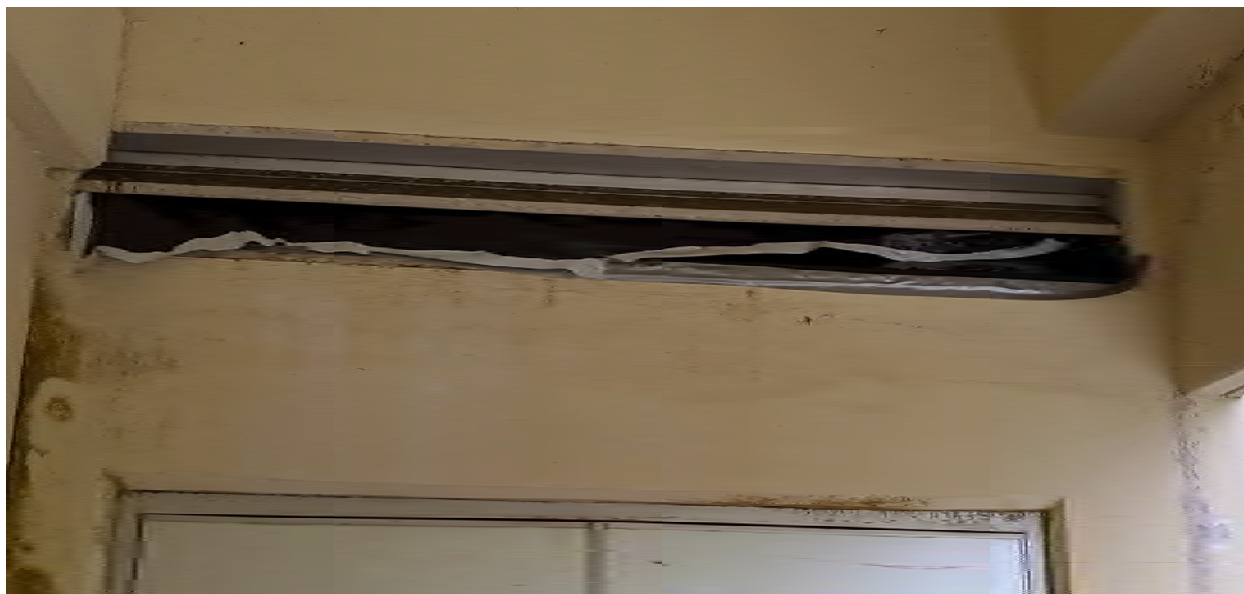
Blocked off outside air intake
