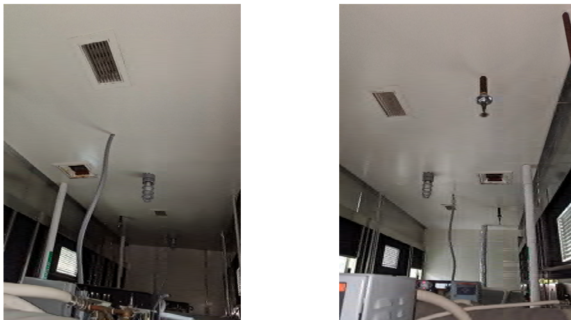
Inadequate exhaust in sterilizer equipment room
