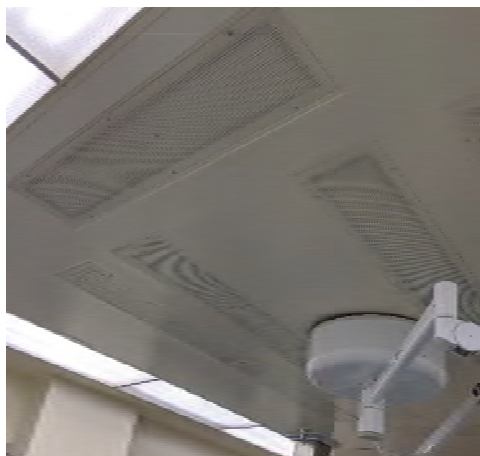
OR ceiling showing inadequate coverage
