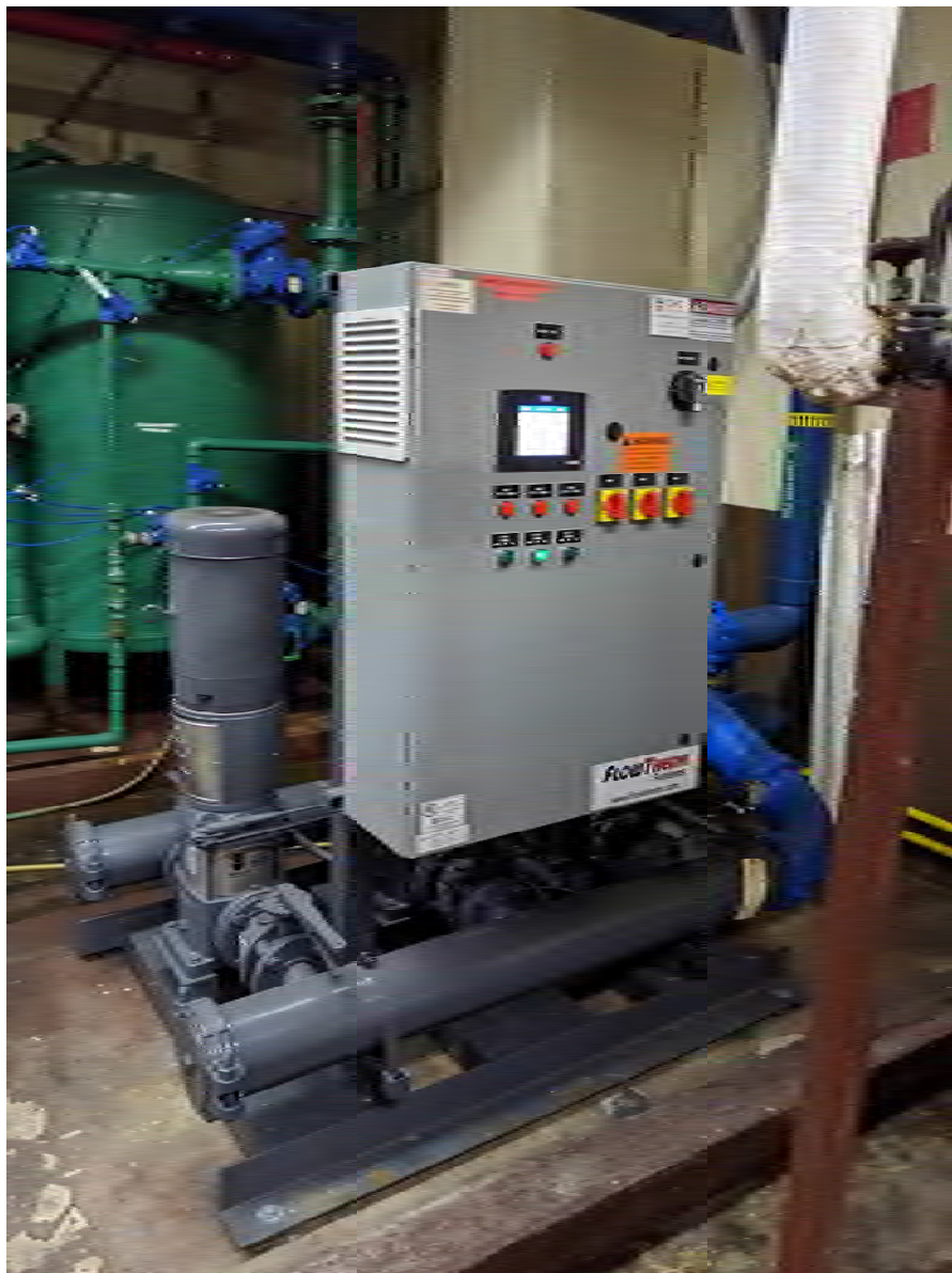
Domestic water pumping unit
