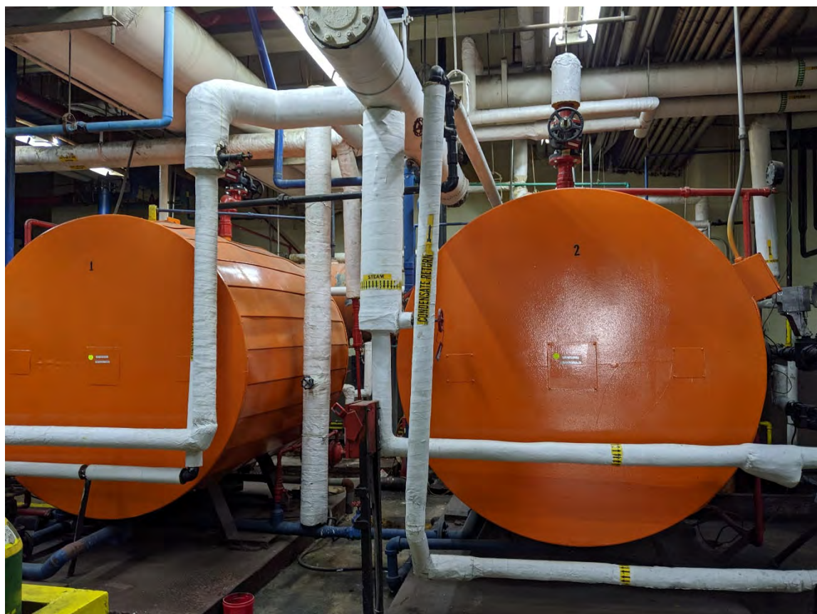
Domestic hot water heat exchangers
