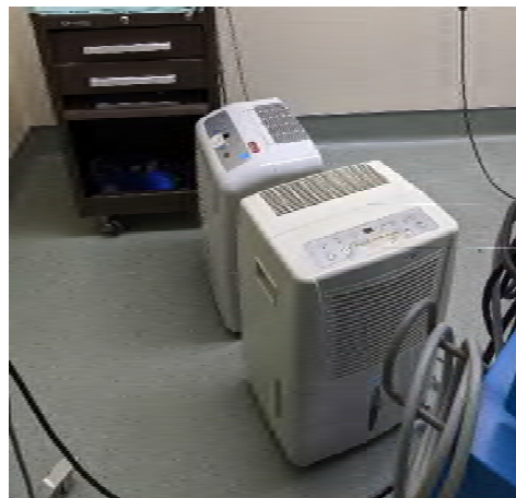
Portable dehumidifiers being used in ORs
