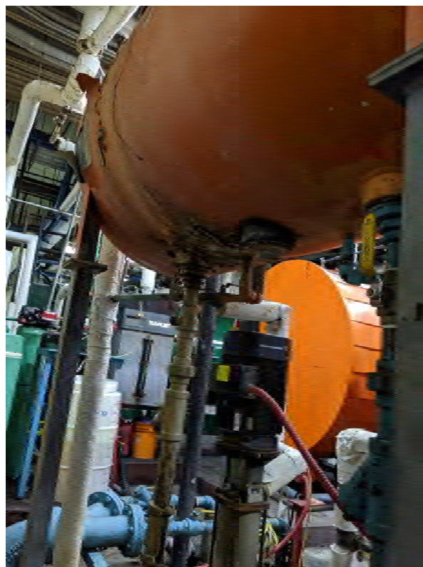
Boiler feedwater/condensate receiver tank
